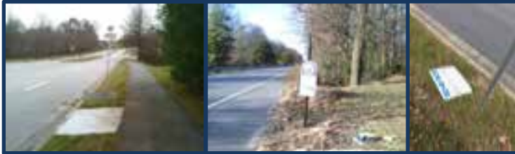
Figure 2-5: Damaged signage. From left, Columbia Gateway & John McAdams, 1257 Ritchie, and Robert
