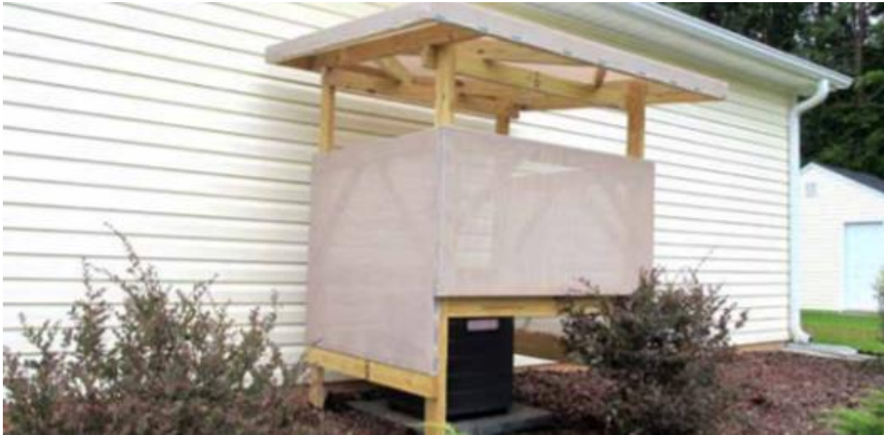
Figure 19. Adjustment to a mechanical equipment capital project to incorporate shading to avoid overheating.
