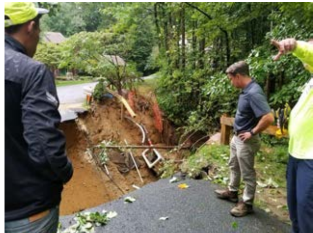
A flash flood in northern Harford County caused major damage to approximately 20 roads and culverts, as streams rose 11 feet above normal water levels on August 31, 2018.
