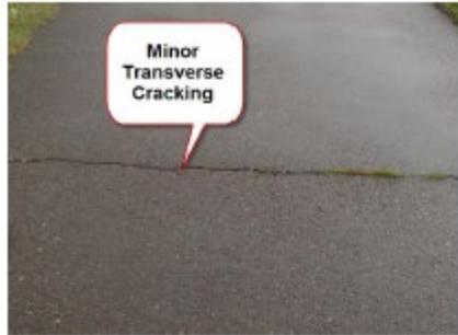
Figure One: Cracking
