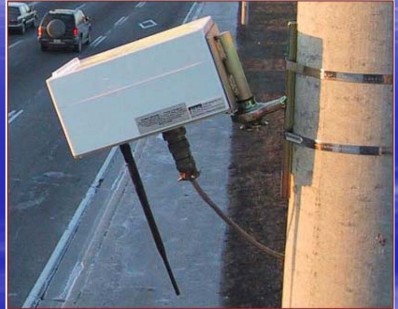
RTMS (Remote Traffic Microwave Sensor) radar
